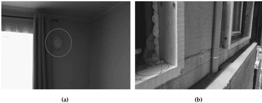
Fig. 13. (a) Supply air valve installed without sector plate and flat ventilation duct inside the insulation layer and (b) ventilation ducts inside the insulation layer.
