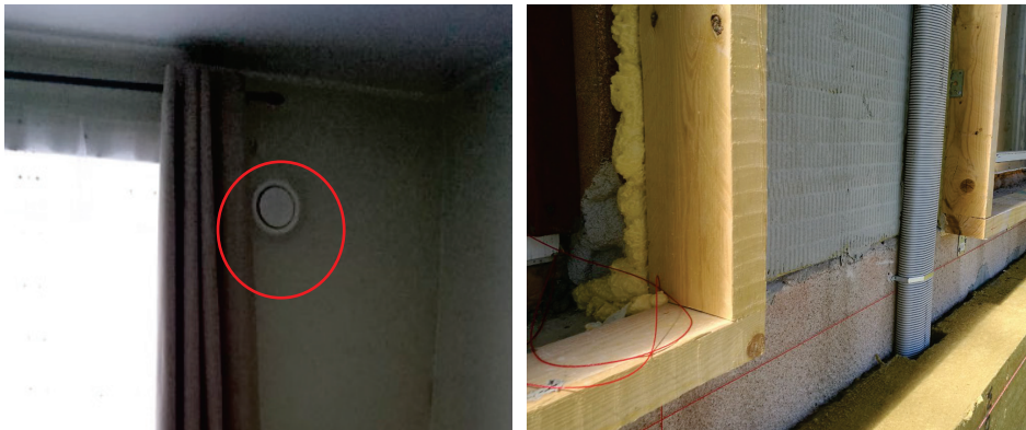
Figure 48. Supply air valve installed without sector plate (left) and apartment ventilation duct inside the insulation layer (right).
