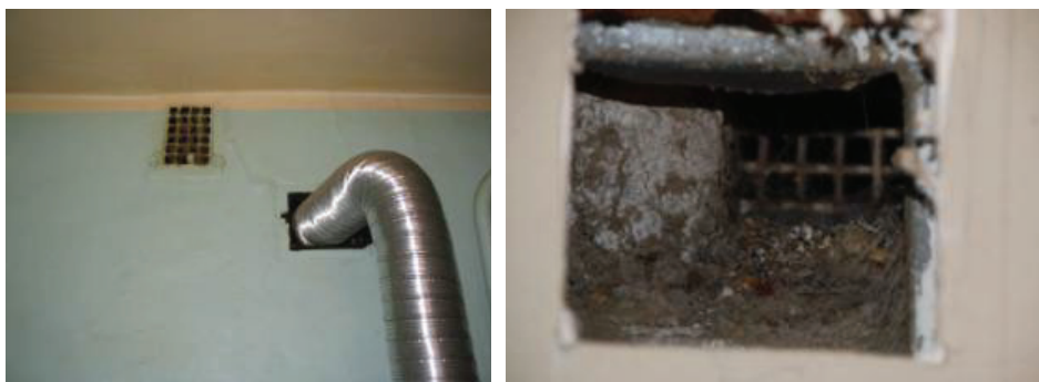
Figure 5. The connection between the old ventilation channels and ductworks of the kitchen hood are not airtight (left) and the dust have accumulated inside the old NV systems (right).
