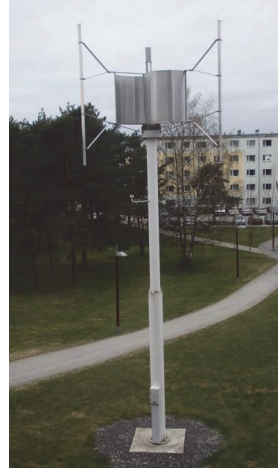
Fig. 13. Prototype generator installed into vertical axis wind turbine.
