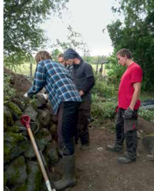
Laur Oberschneider is conducting students' fieldwork in order to repair the back corners of the cellar's dry walls. Photo by Malvo Tominga.
