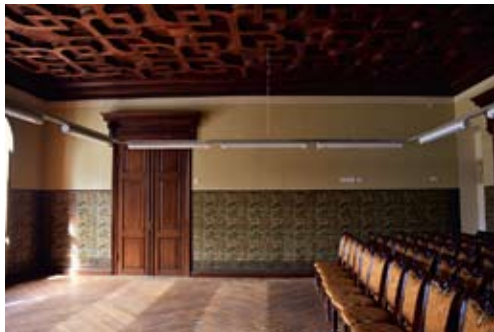
Figure 119. Final outcome of the papered room. Historic unity is broken by unfitting modern lights.
