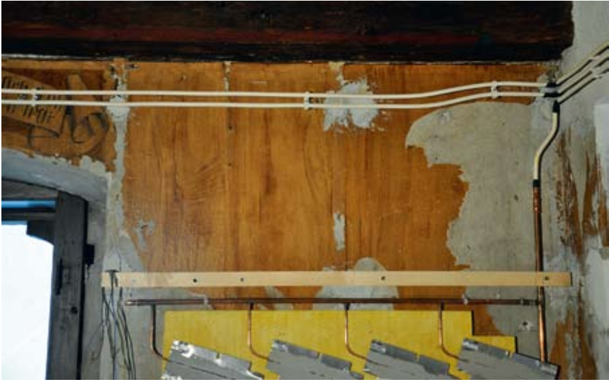
Figure 103. If damaged wallpapers are not planned to be exhibited, they should not be retouched.
