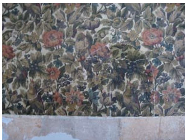
Figure 95. Large missing areas in the wallpaper were filled with fragments found behind the overdoors of the dining-room of the Puurmani manor.
