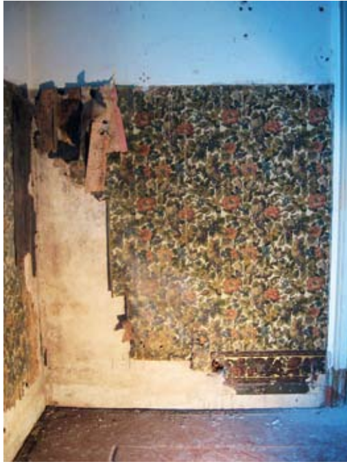
Figure 114. Corner of the dining-room badly damaged by humidity and mould.
