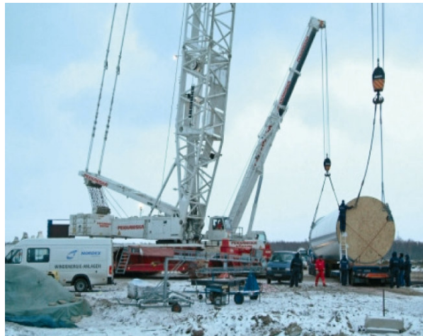
Joonis 2. Tuuliku monteerimine Pakri poolsaarel Figure 2. Erection of a wind turbine on the Pakri peninsula
