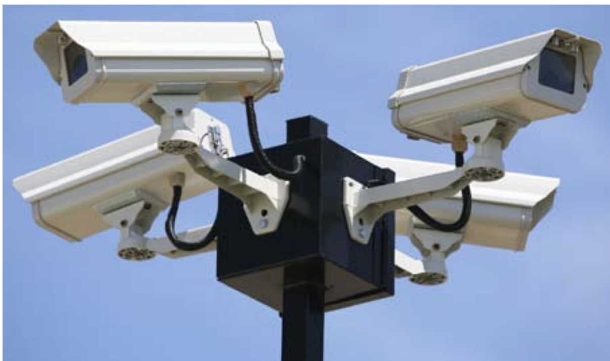
Closed circuit television (CCTV) must be used responsibly and with effective safeguards in place.
