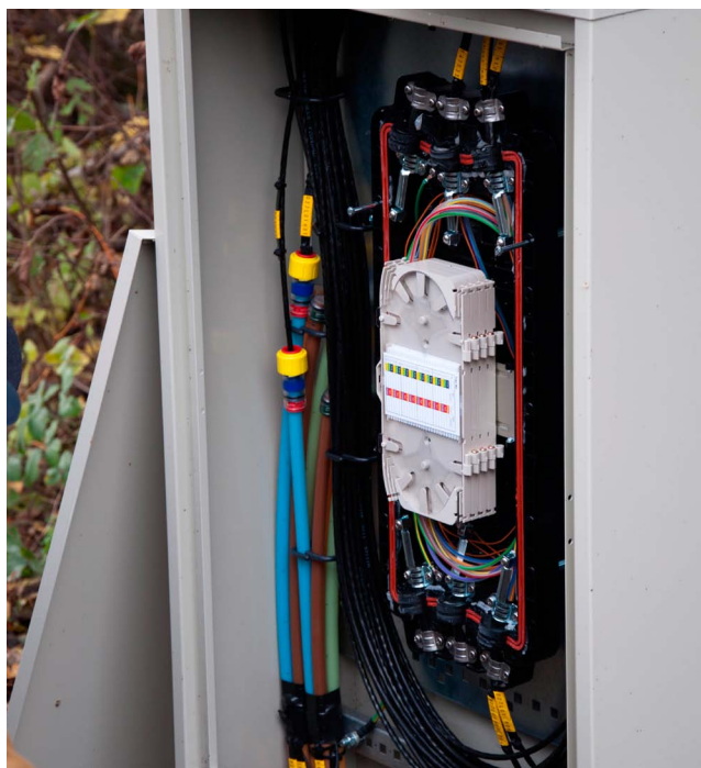
EstWin fiber optic cables
